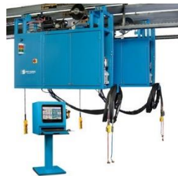
DataFill A/C Fill System with VF Drives
