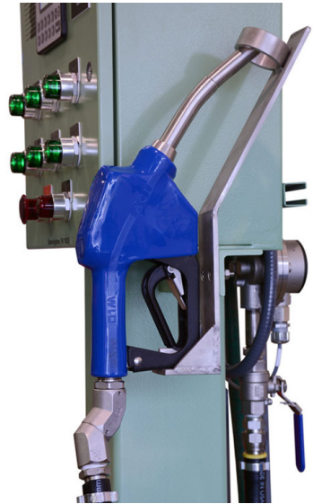
DEF Fill Station and Nozzle
